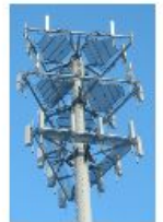
Wireless Communications Base Stations
