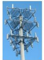
Wireless Communications Base Stations
